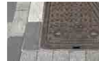
Access cover integrated into paving with minimal infill
