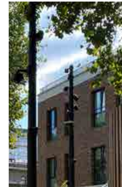
Light column with multiple spotlights and CCTV attached
